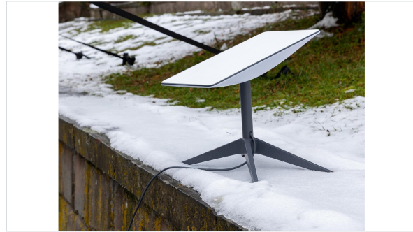
FIG. 2 | Starlink ground terminal installed outdoors.
